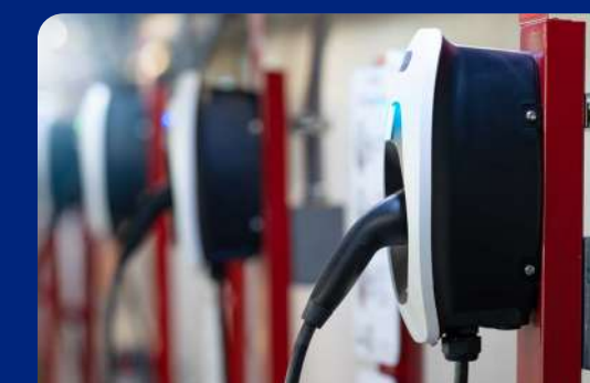
EV charger network creation
